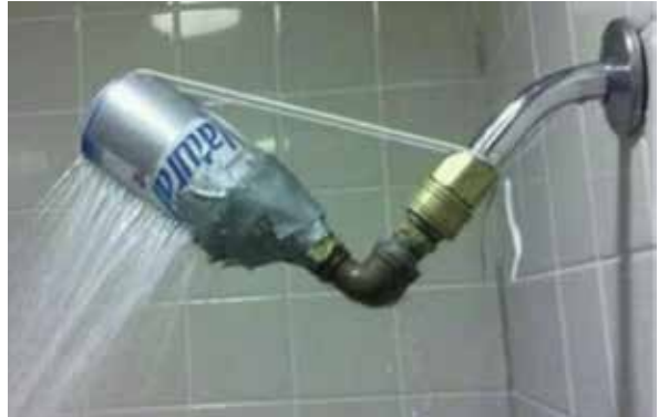
Shower head need replacing?
